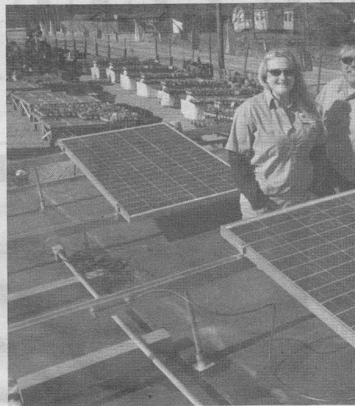
Michelle Harvey and Mark Bursch of Lakeview Nurseries standing on a roof with solar panels being installed.
